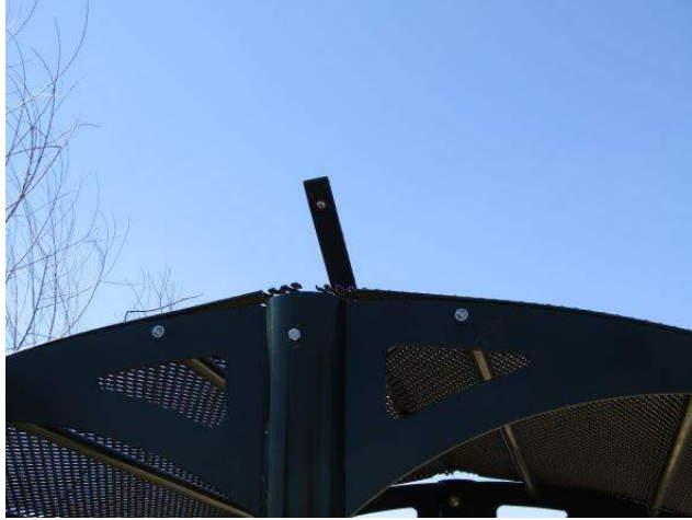
Shade Bench Bracket needs to be secured
