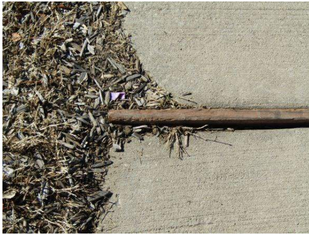
Sidewalk spacer creating trip hazard
