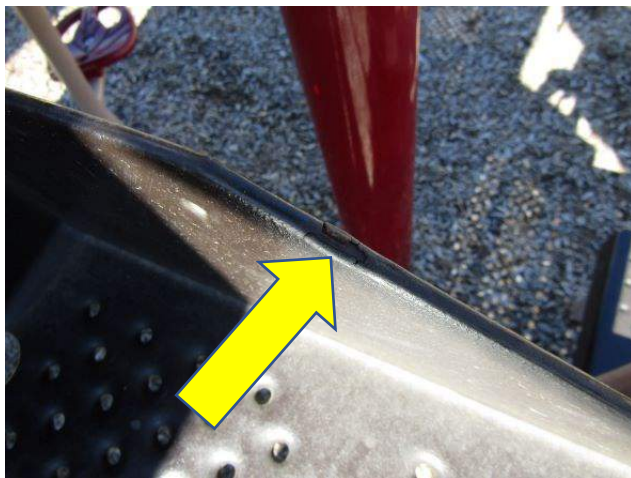
MINOR PVC damage transfer station steps
