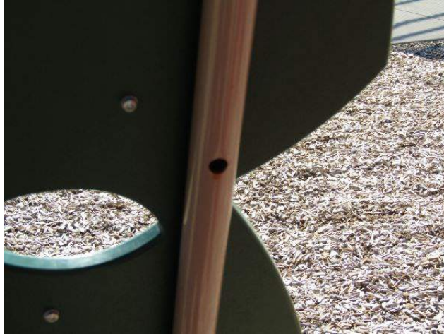
Missing bolt on Wall Climber (Replaced during inspection)
