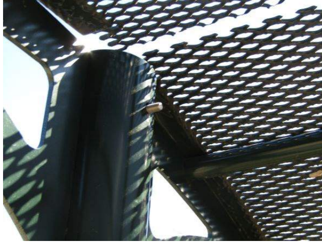
Missing nut for bolt
