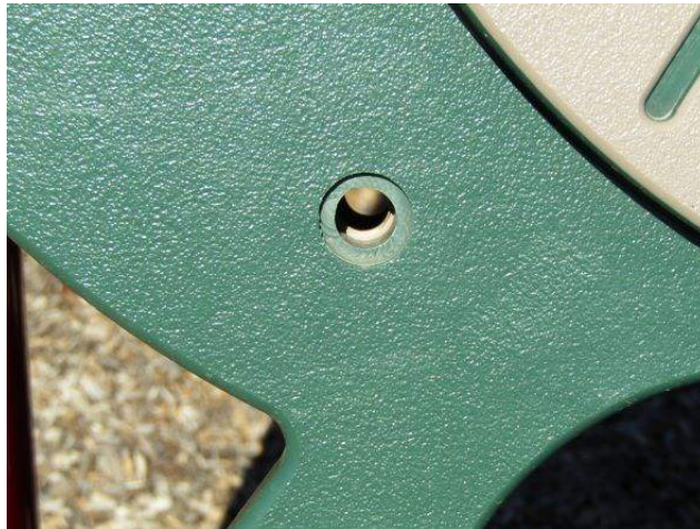
Same missing bolt as above (Frontside)
